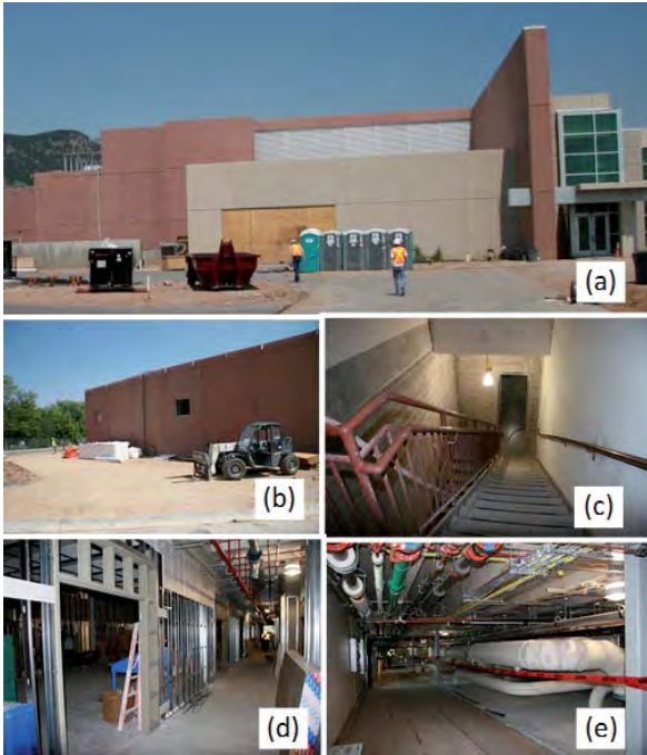
Figure 8. Building 87: (a) the south exterior, (b) the north exterior, (c) the main stairwell, (d) the interior wall construction, and (e) some of the extensive mechanical piping found throughout the building.
