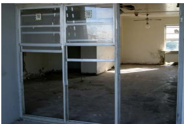
Figure 1c. An interior view of the 13-story apartment building in New Orleans, Louisiana.
