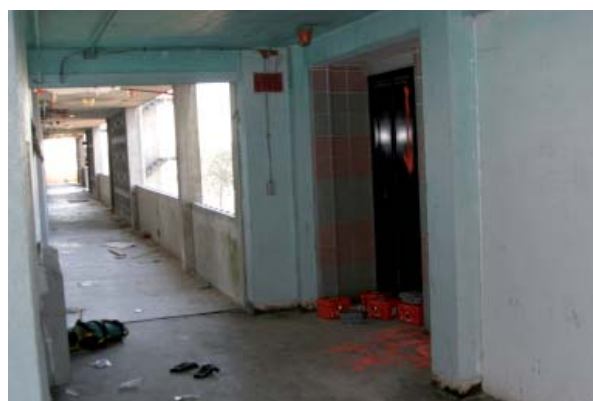
Figure 1d. An interior view of the 13-story apartment building in New Orleans, Louisiana.
