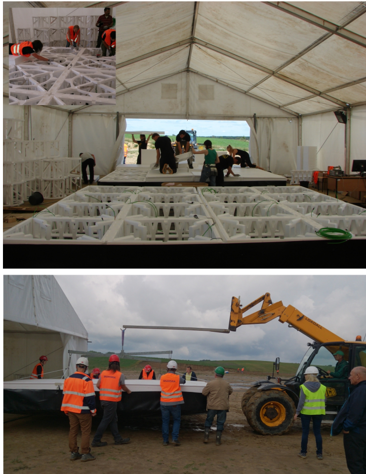
Figure 3. The process of assembling of HBA antennas and transporting ready tiles to the right place at the field. In both activities the huge roles were played by students.
