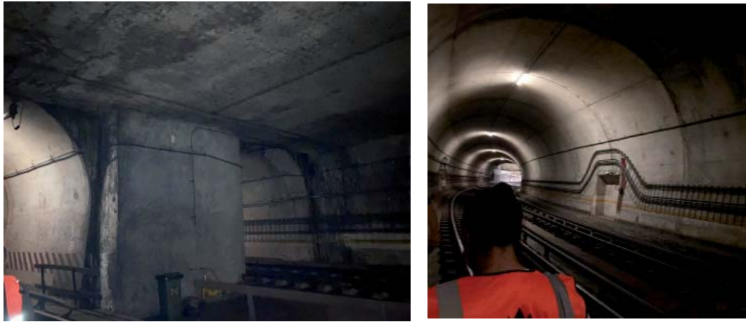
Figure 5. Photo of the bifurcation at "Carnide" station (a), and oval tunnel (b).
