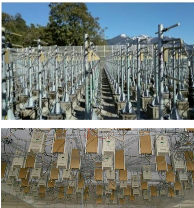
Figure 1. (a) The antenna array on the rooftop and (b) the transmitting/receiving modules hanging from the ceiling of the floor below.
