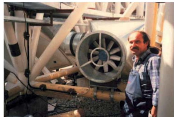
Figure 15b. One of the five ventilators that cause a circulating air movement with controlled temperature through the backup structure. This structure is covered on the outside by a cladding of thermal insulation panels, visible in the upper picture.
