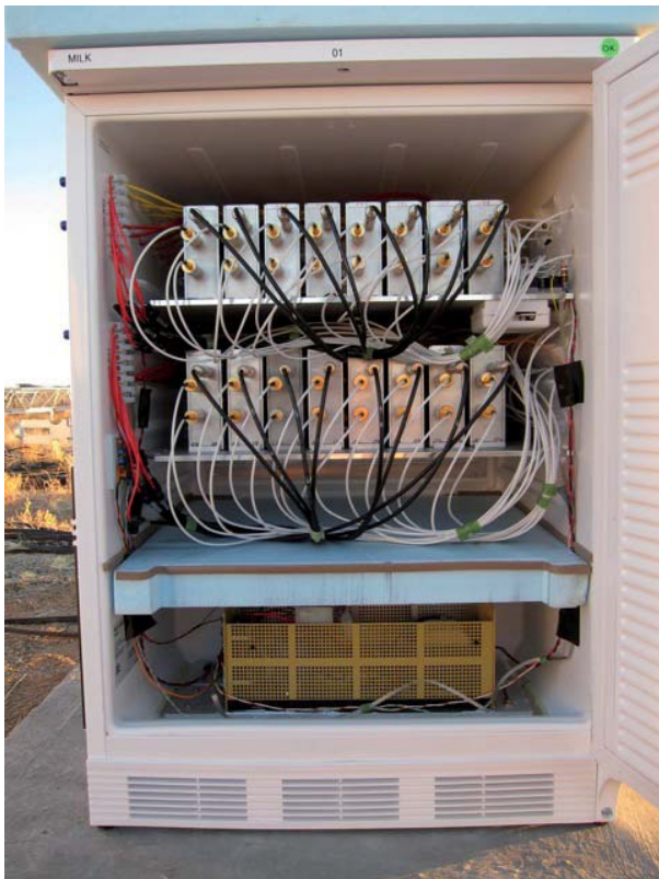
Figure 13. The enclosure housing 16 receiver modules. It is shown here residing on its concrete pad in The Karoo.
